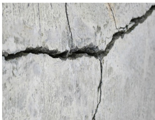
© stone crack, Fotolia #3669926
